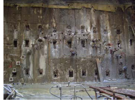
Fig 3: Top half of one of the galleries before excavation. All boreholes in this section have been drilled except for five on the far left hand side, which are marked by square steel plates. The location of the sacrificial bore can just be seen in the centre of the gallery, about 1.5m beneath the highest borehole.
