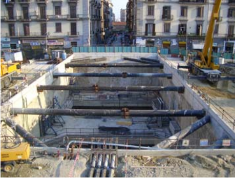
Fig 2: Overview of the location. Here you can see the large steel beams supporting the inner walls.
