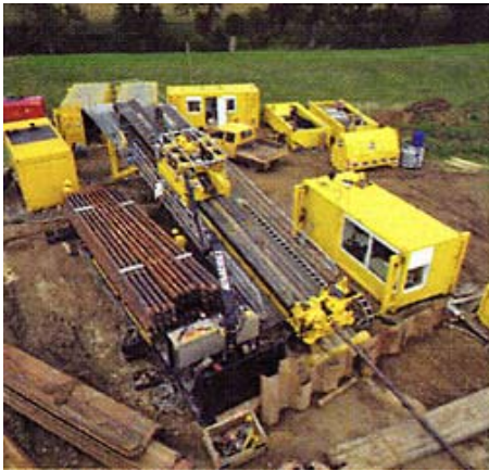
Haustadt & Timmerman used its new 400 ton (360-m-ton) Herrenknecht rig for part of this job.
